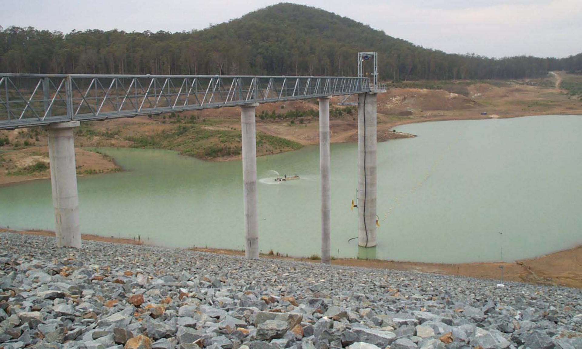
Submerged Aeration System & Mixer Units on Intake Tower
